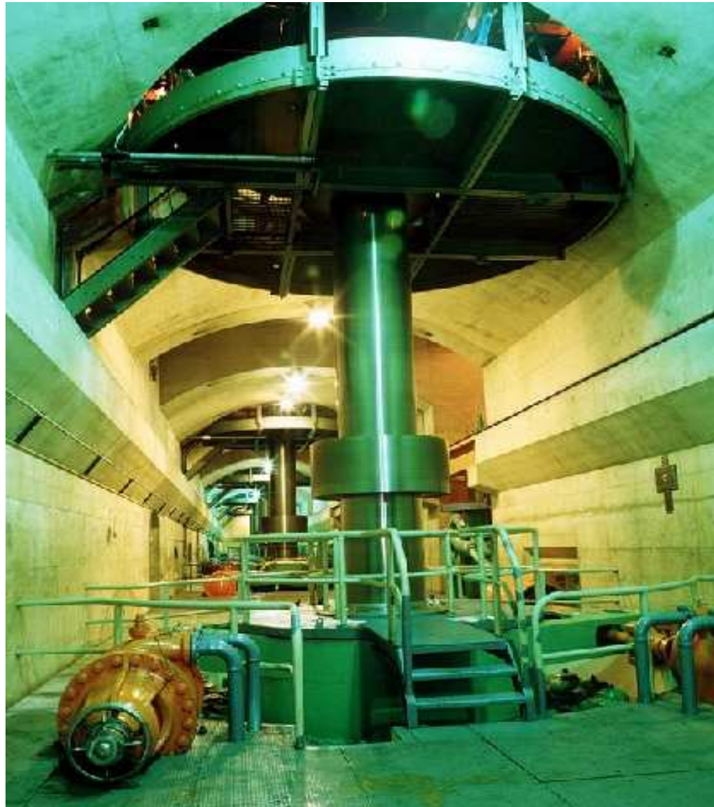
The shaft that connects the turbine and generator
